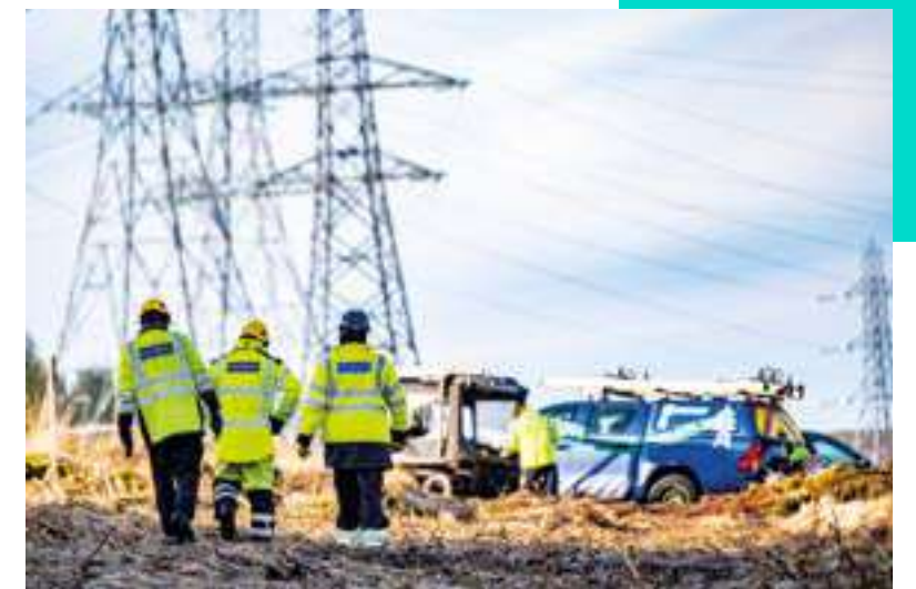
Management of risk is key to delivery of SSE's Large Capital Projects
