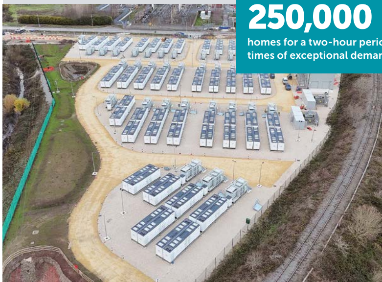
From coal to battery storage – Ferrybridge is providing the flexible power of the future
