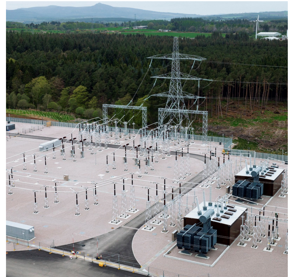
SSEN Transmission Kintore Substation
