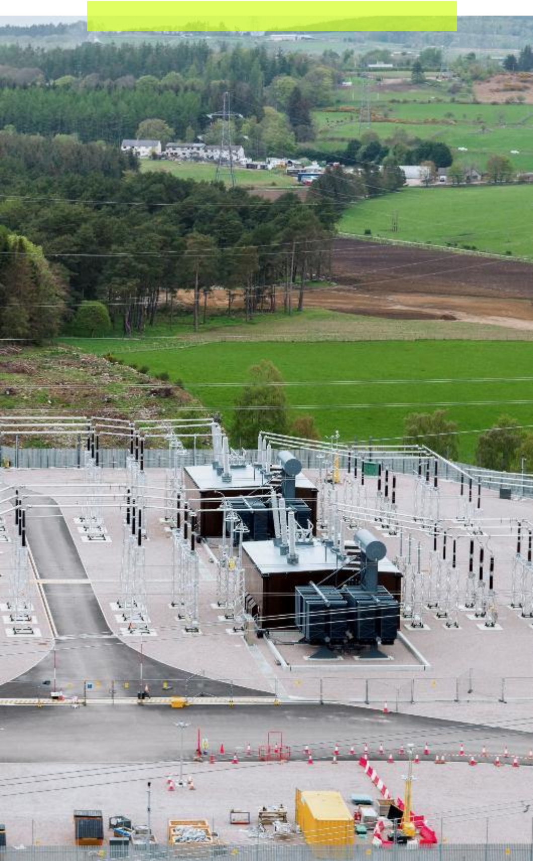
Kintore 400kV Substation
